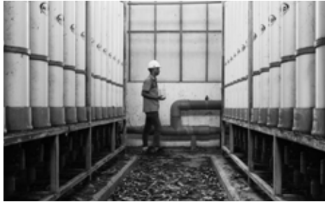
Indonesia-D AGUNG KRISPRIMANDOYO-water treatment plant
