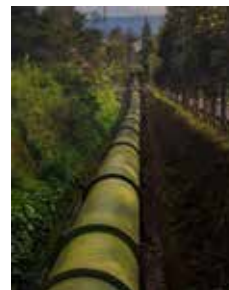
Indonesia-YURI REVALINO- Wonosobo hydropower giant pipe
