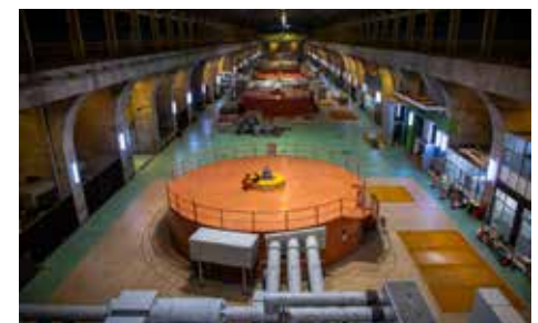
Indonesia-deden iman-Cirata Hydroelectric Power Plant
